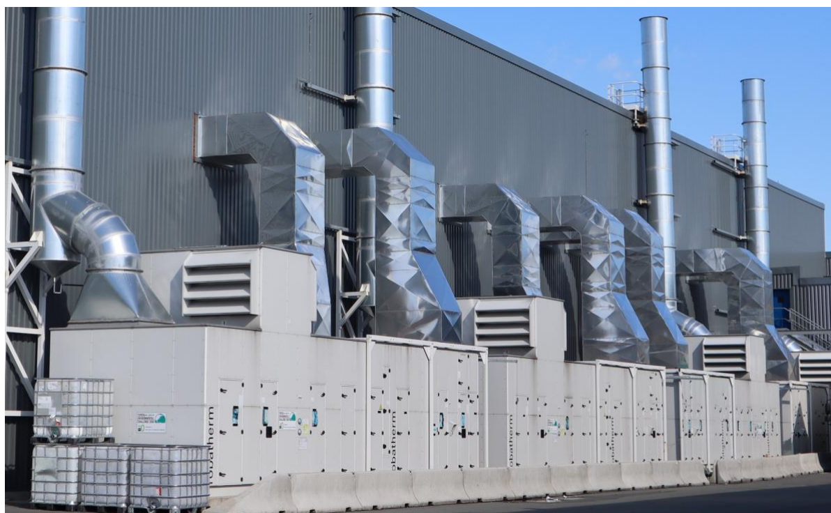
Figure 1 Carbon-free Air Handling Unit for Paint Process of plastic parts at Toyota's plant in France. Toyota uses Meteomatics data to understand energy consumption of Air Handling Units for buildings and processes.
